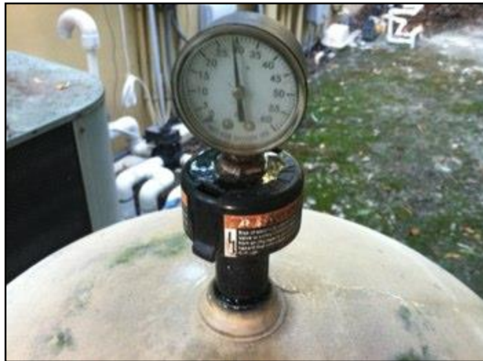
Leaking Pressure Gauge
