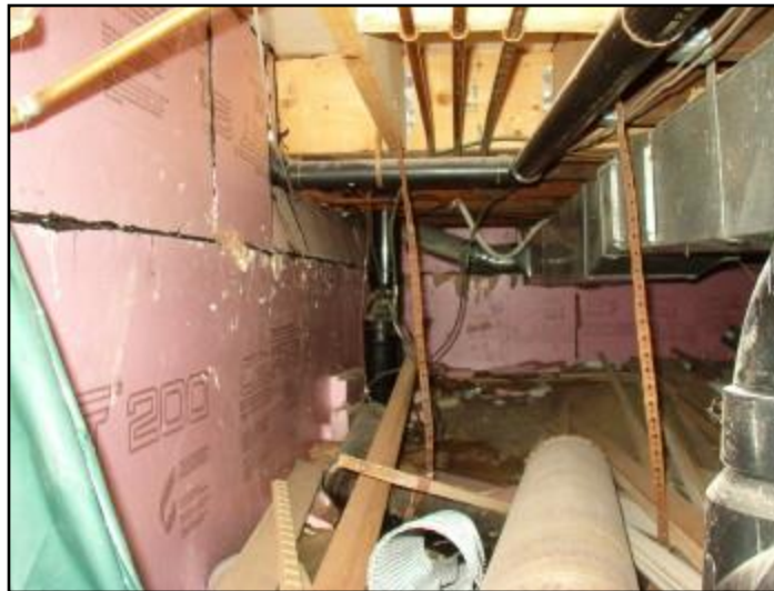
12. Exposed polystyrene insulation is fire hazard
