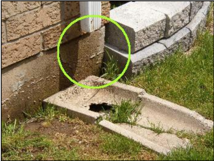
3. Downspout ends too close to building
