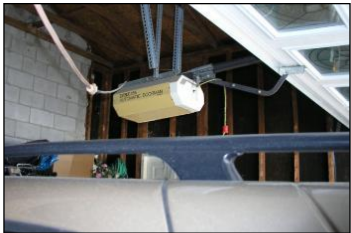
17. Extension cord for west garage door opener
