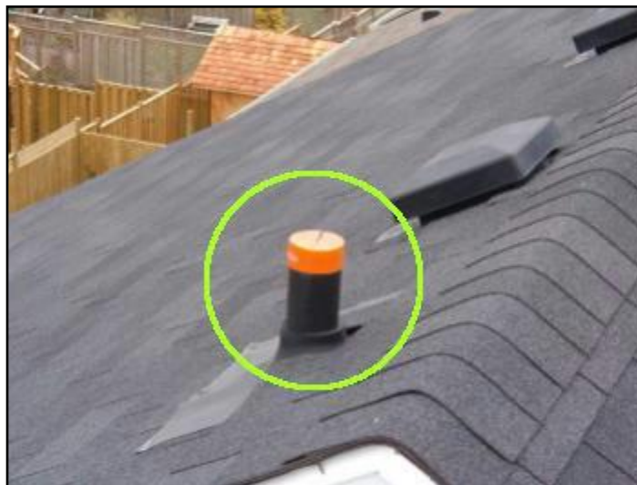
15. Plumbing stack is capped
