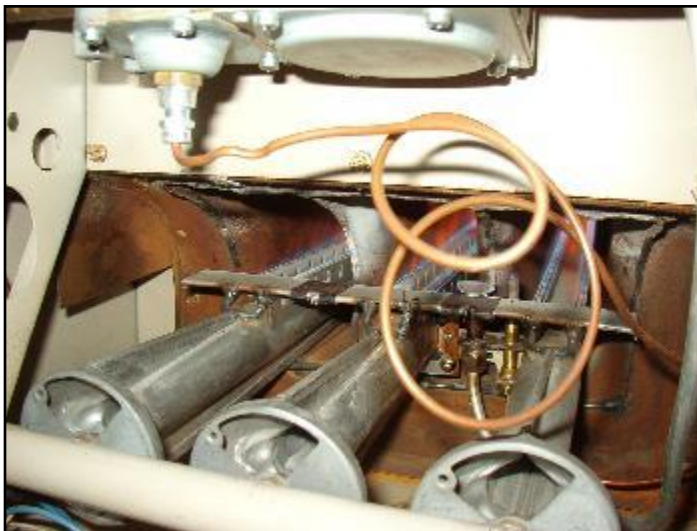
9. Rust at bottom of heat exchanger
