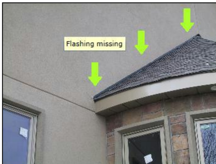
1. No kickout flashing at roof/sidewall junction
