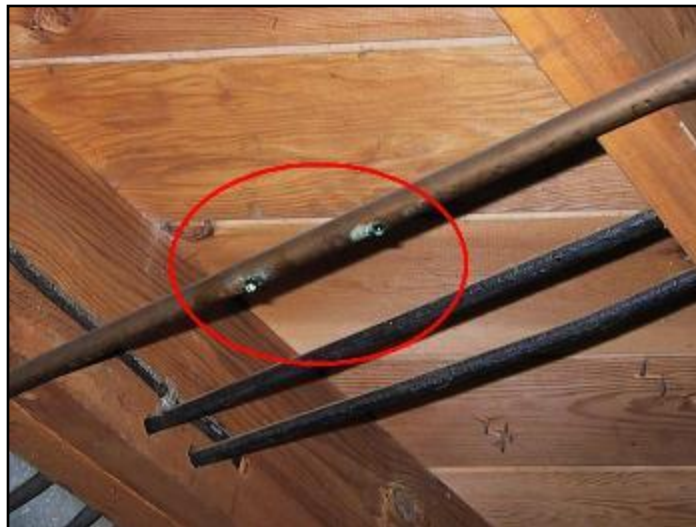
13. Leaking copper supply pipe
