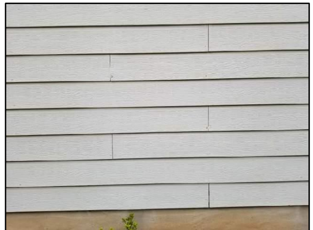
5. Siding runs right to horizontal flashings—a...
