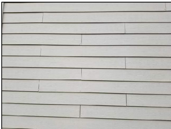
18. Siding runs right to horizontal flashings—a...
