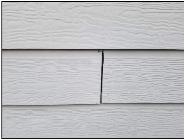
2. Siding runs right to horizontal flashings—a...
