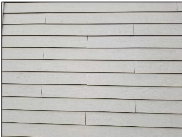
4. Siding runs right to horizontal flashings—a...
