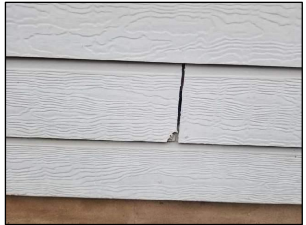
3. Siding runs right to horizontal flashings—a...
