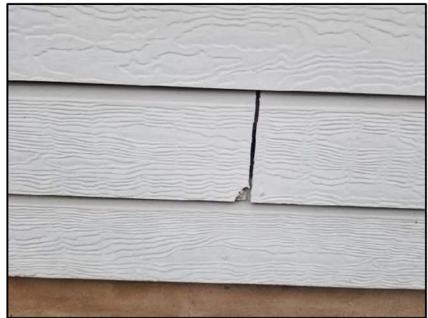
17. Siding runs right to horizontal flashings—a...
