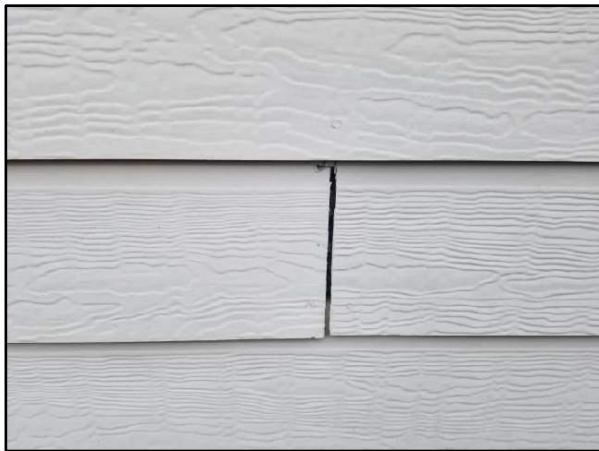
16. Siding runs right to horizontal flashings—a...
