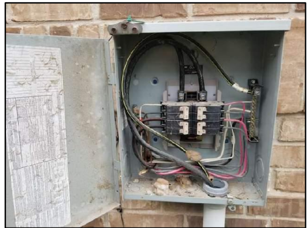
24. Breakers - exterior wall
