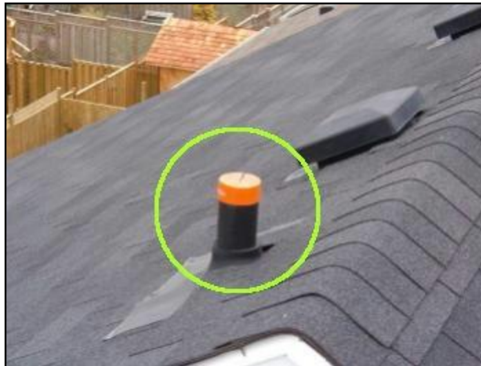
Plumbing stack is capped
