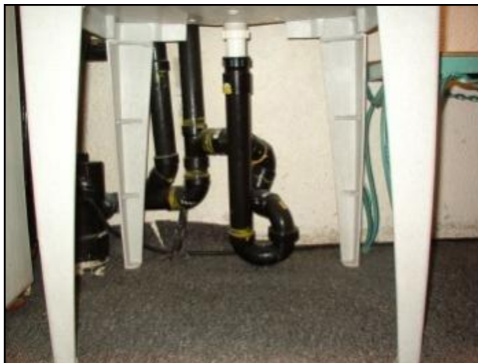
Poor trap arrangement
