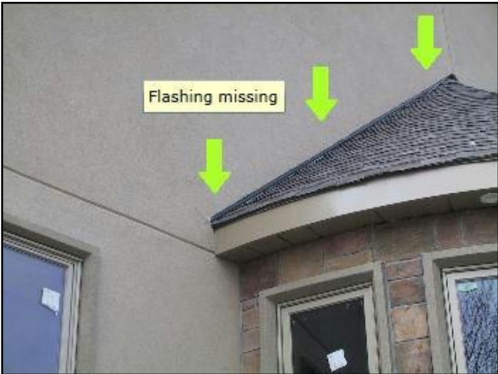
No kickout flashing at roof/sidewall junction
