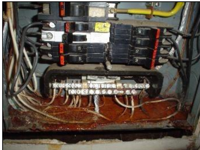
Water and rust in bottom of panel
