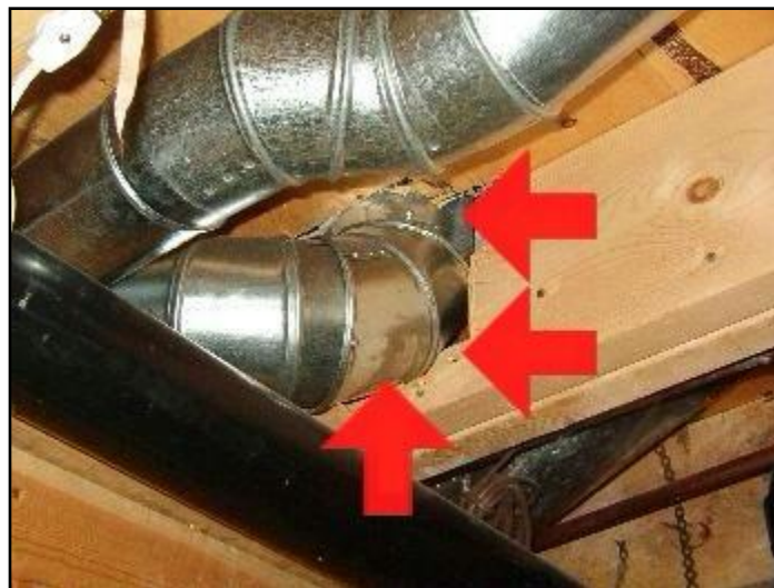
Joists are notched and weakened
