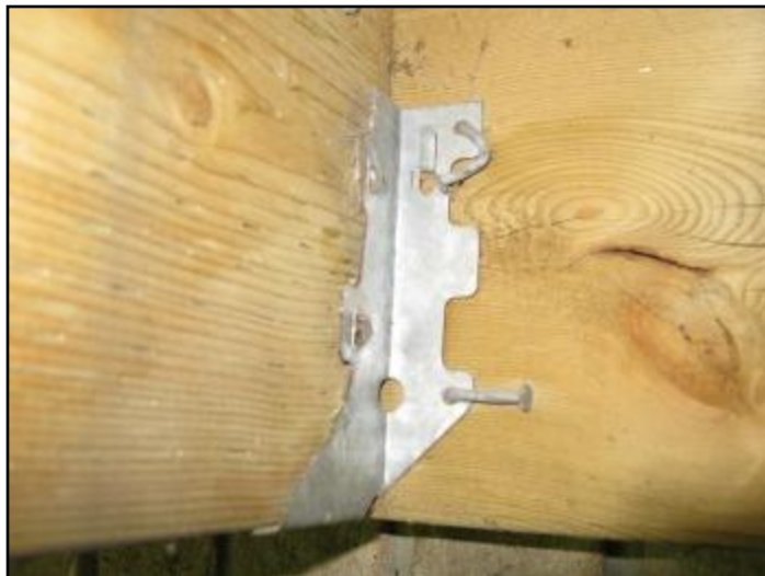
Poor end bearing, joist hanger connections
