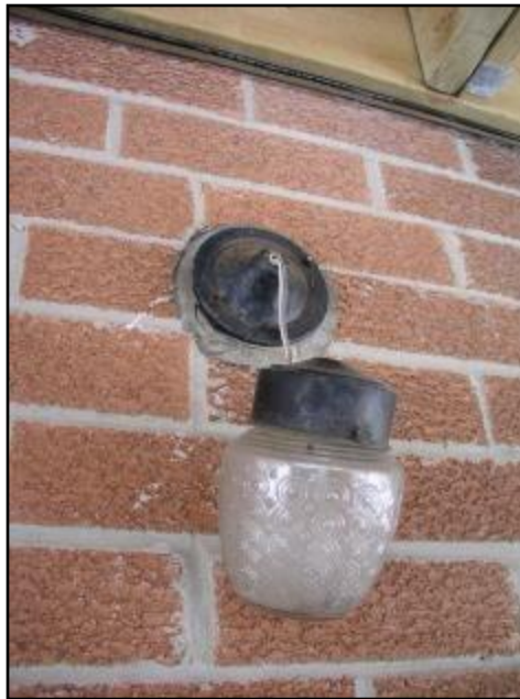
Light fixture is not well secured
