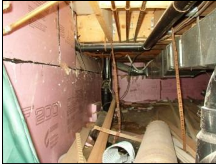
Exposed combustible insulation
