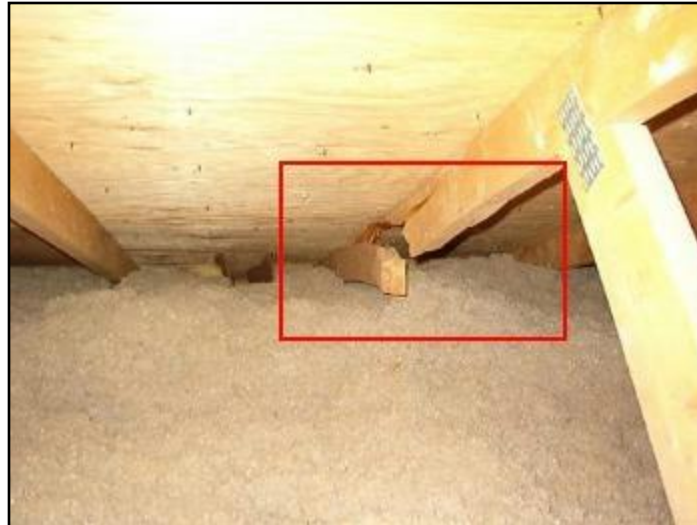
Top chord of truss is split
