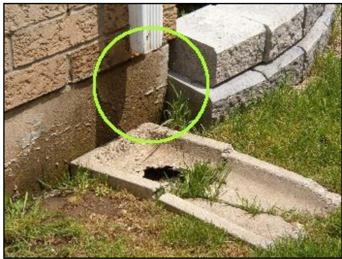
Downspouts discharge too close to building
