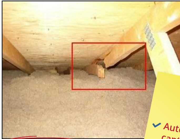
Top chord of truss is split
