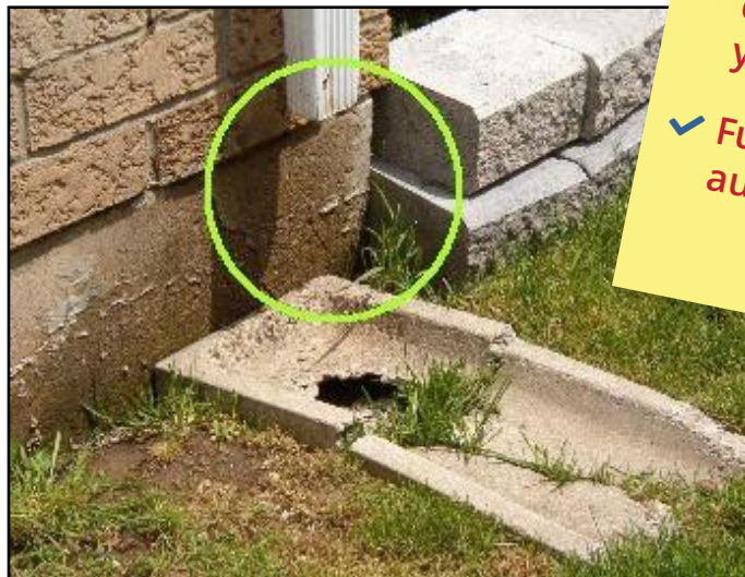
Downspouts discharge too close to building
