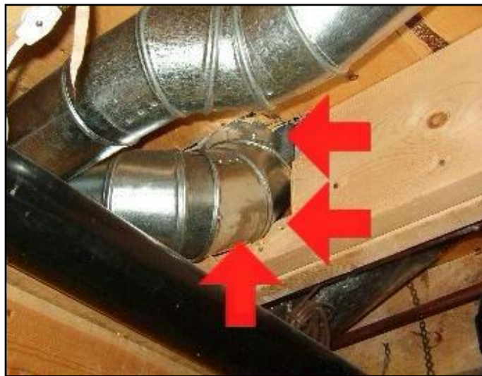
Joists are notched and weakened
