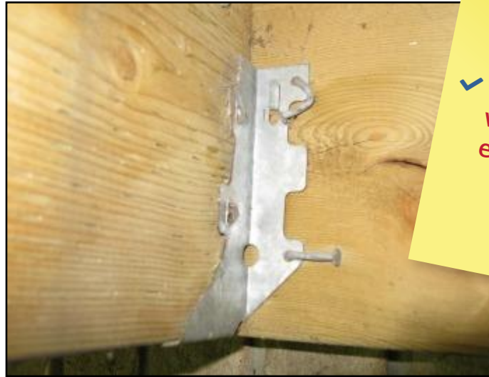
Poor end bearing, joist hanger connections
