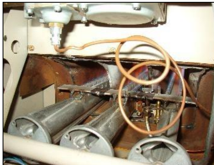
Draft hood spillage or backdraft
