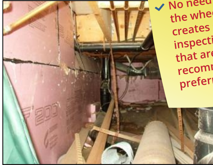
Exposed combustible insulation
