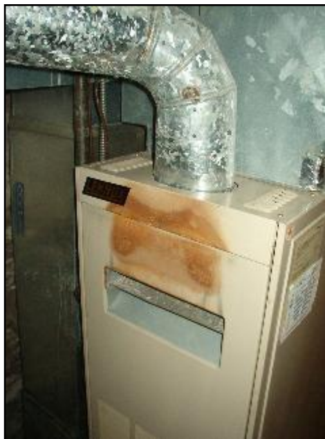
Draft hood spillage or backdraft
