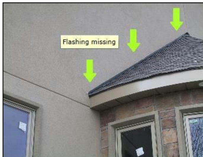
No kickout flashing at roof/sidewall junction
