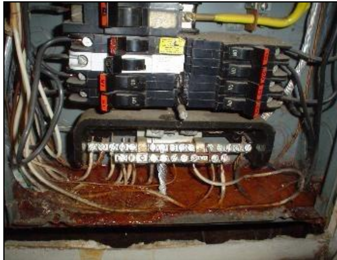
Water and rust in bottom of panel
