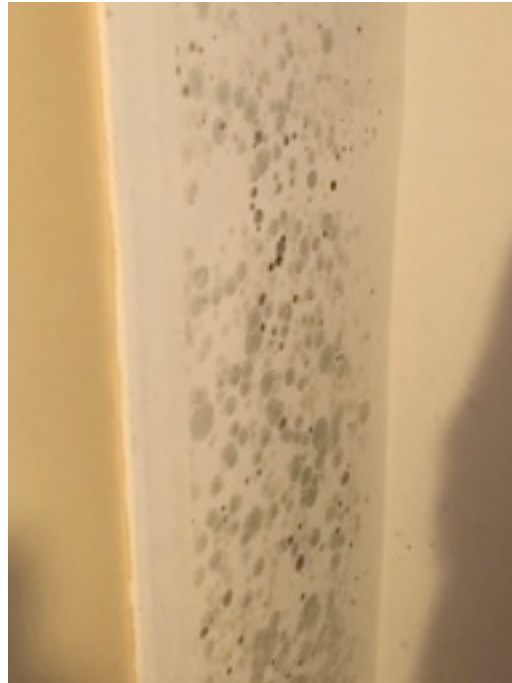
Photo 3: Mould growth noted inside the closet of Bedroom 2.
