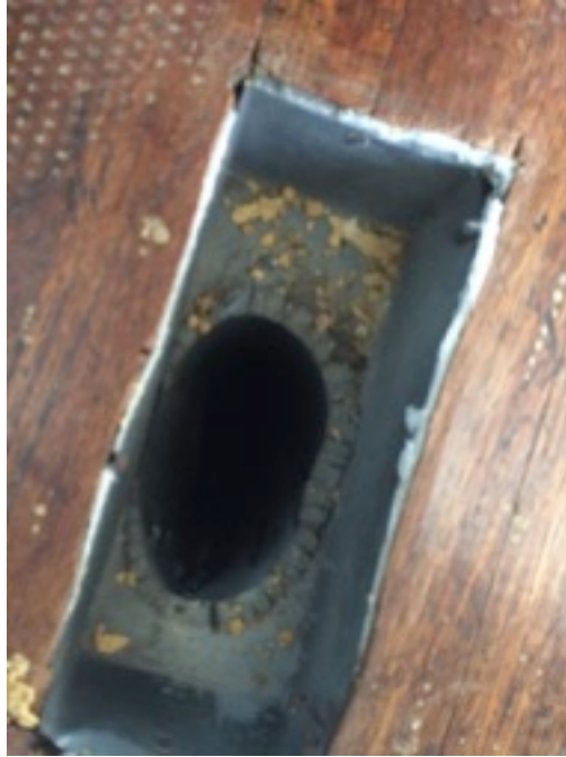
Photo 7: Asbestos-containing duct paper insulation insulating supply air ducts throughout the home.
