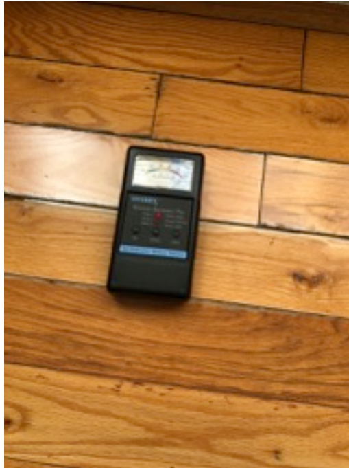
Photo 1: Elevated moisture readings on the flooring of the Master Bedroom.
