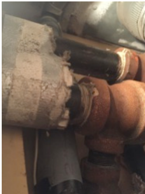
Photo 6: Asbestos pipe insulation noted in poor condition.
