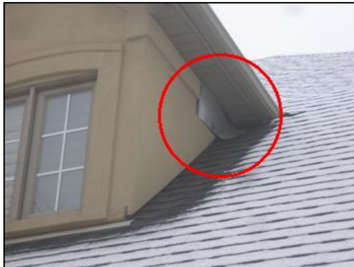
proper repairs needed
