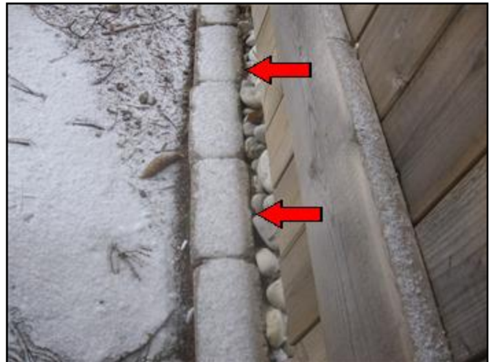
small retaining wall is bowing, leaning
