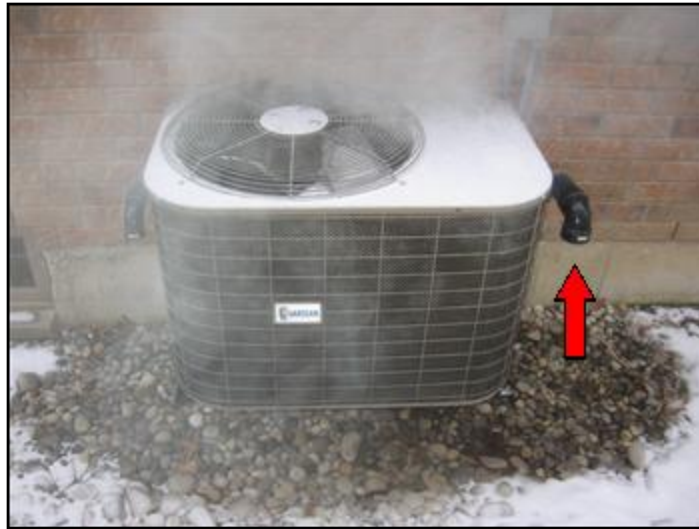
water hater discharge too close
