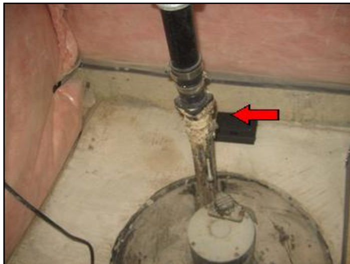
previous leakage noted
