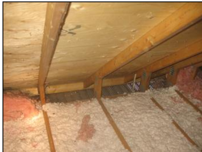
insulation missing (removed) at soffit
