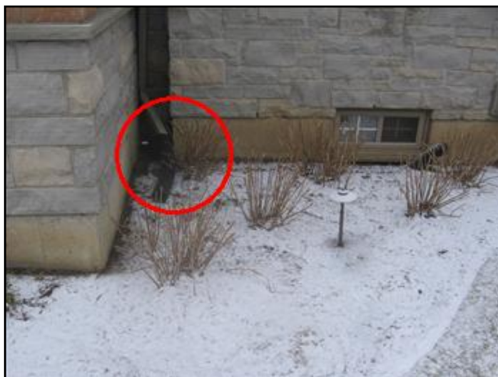
downspout empties at low area
