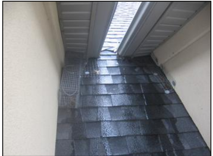
vermin screens at rear soffit
