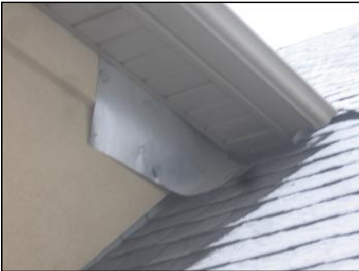
crude patch job at front dormer- entry site?
