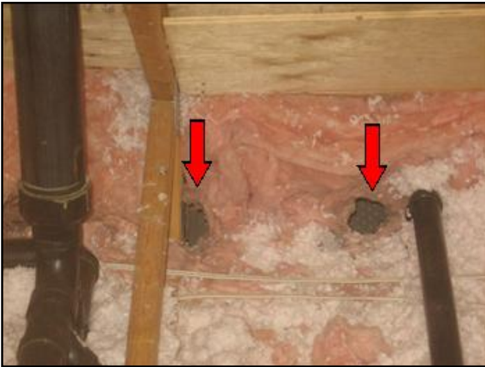
holes through insulation in soffit
