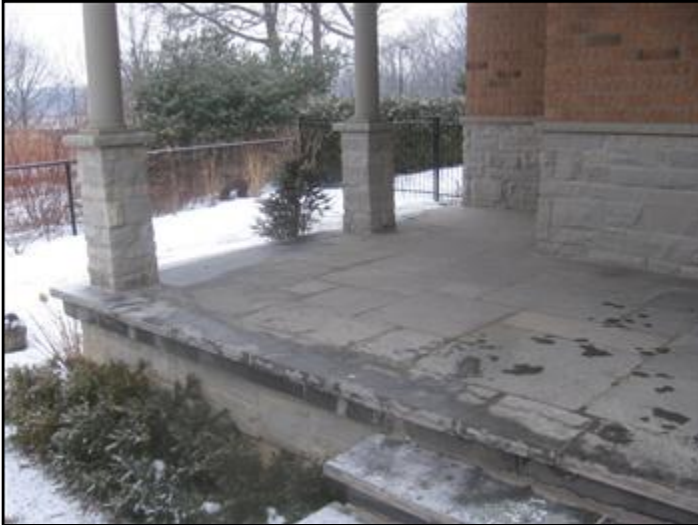
no handrail- fall hazard
